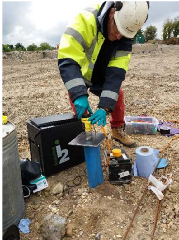
Figure 4. An Ecologia employee installing the device. The system is set up using a laptop computer, and then runs from a 12V battery.
