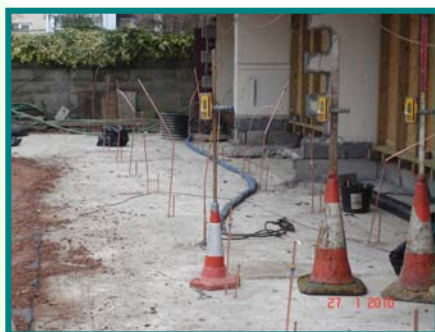
Injection of Uretek low density resin into void space under ground bearing slab
