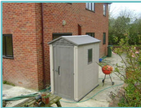
Water heater located within a small shed in the rear garden of the domestic property.
