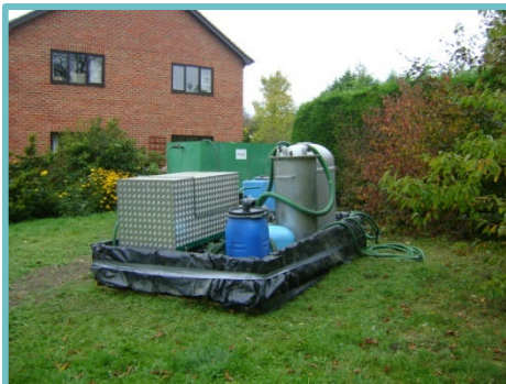
Multiphase extraction system located outside the property.
