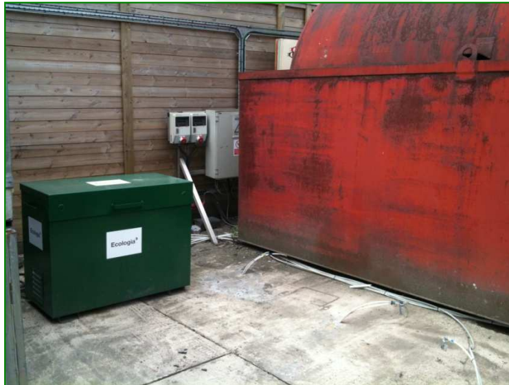
Sparging system during operation
