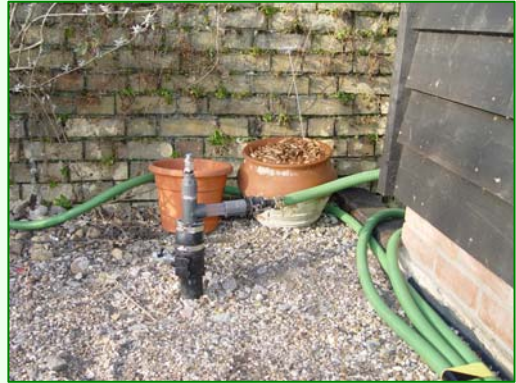
Typical ECOVAC dual phase extraction well
