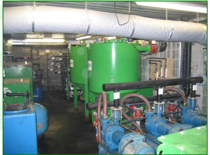
The remediation equipment was located in a cellar under the new development
