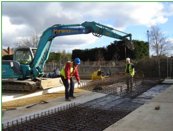
Re-instatement of a section of hardstanding after installation Of Horizontal extraction and injection pipes
