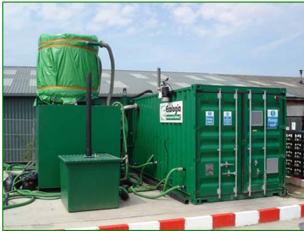
The remediation system, designed and manufactured by Ecologia in Kent
