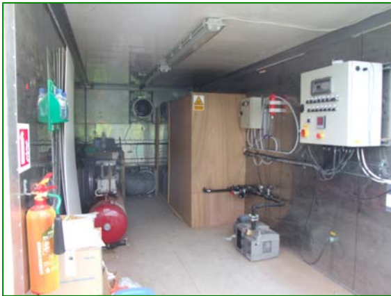
Internal view of the Ozone Unit
